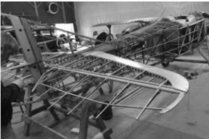
The complexity of the tail was just a preview of the complexity throughout the rest of the airplane. The woodwork on this airplane is the most challenging of any tackled by the GAAM volunteers.
